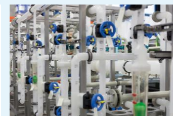
Flow instrumentation and measurement
